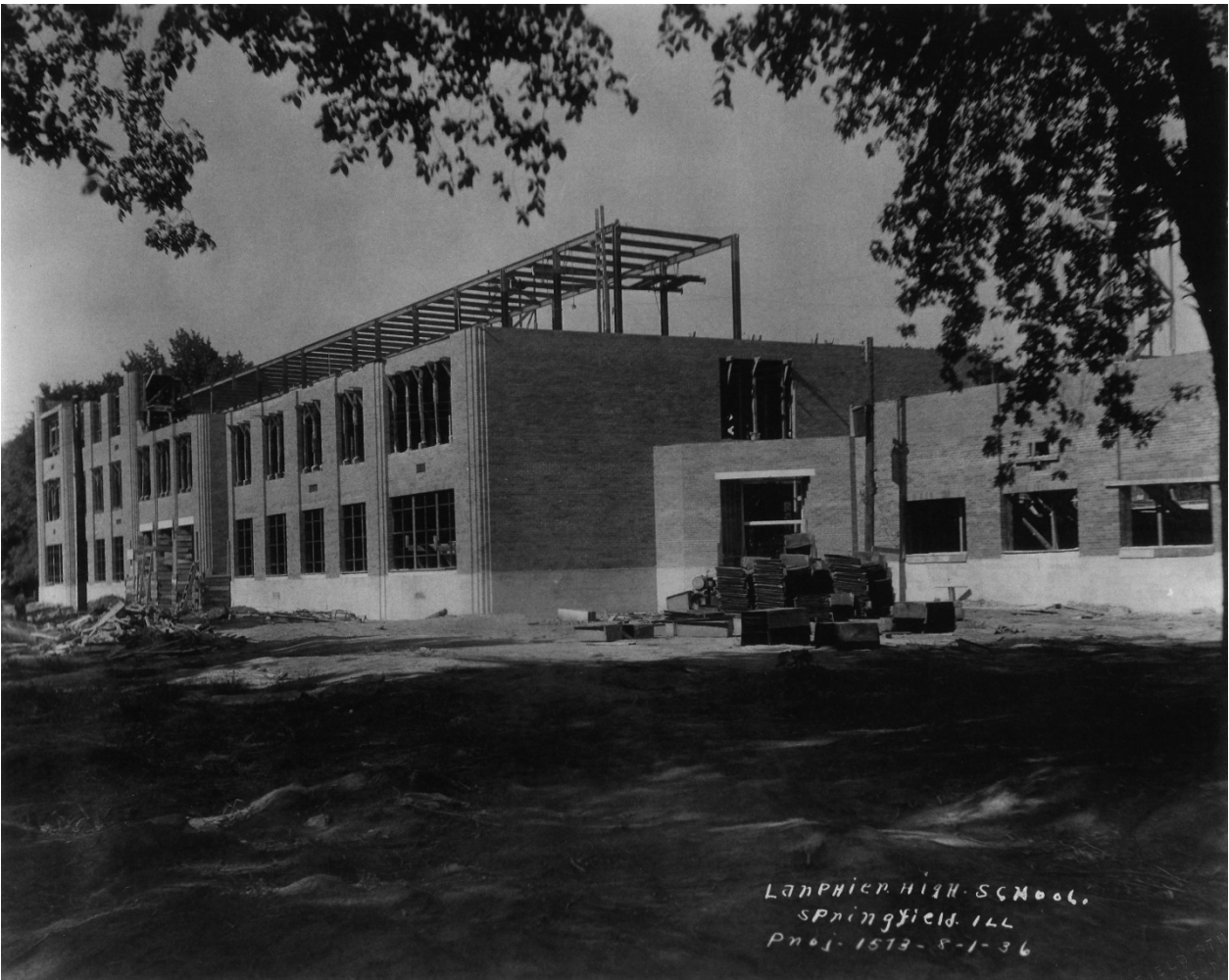
Lanphier High School construction, August 1, 1936. Photo courtesy Sangamon Valley Collection Lincoln Library.
