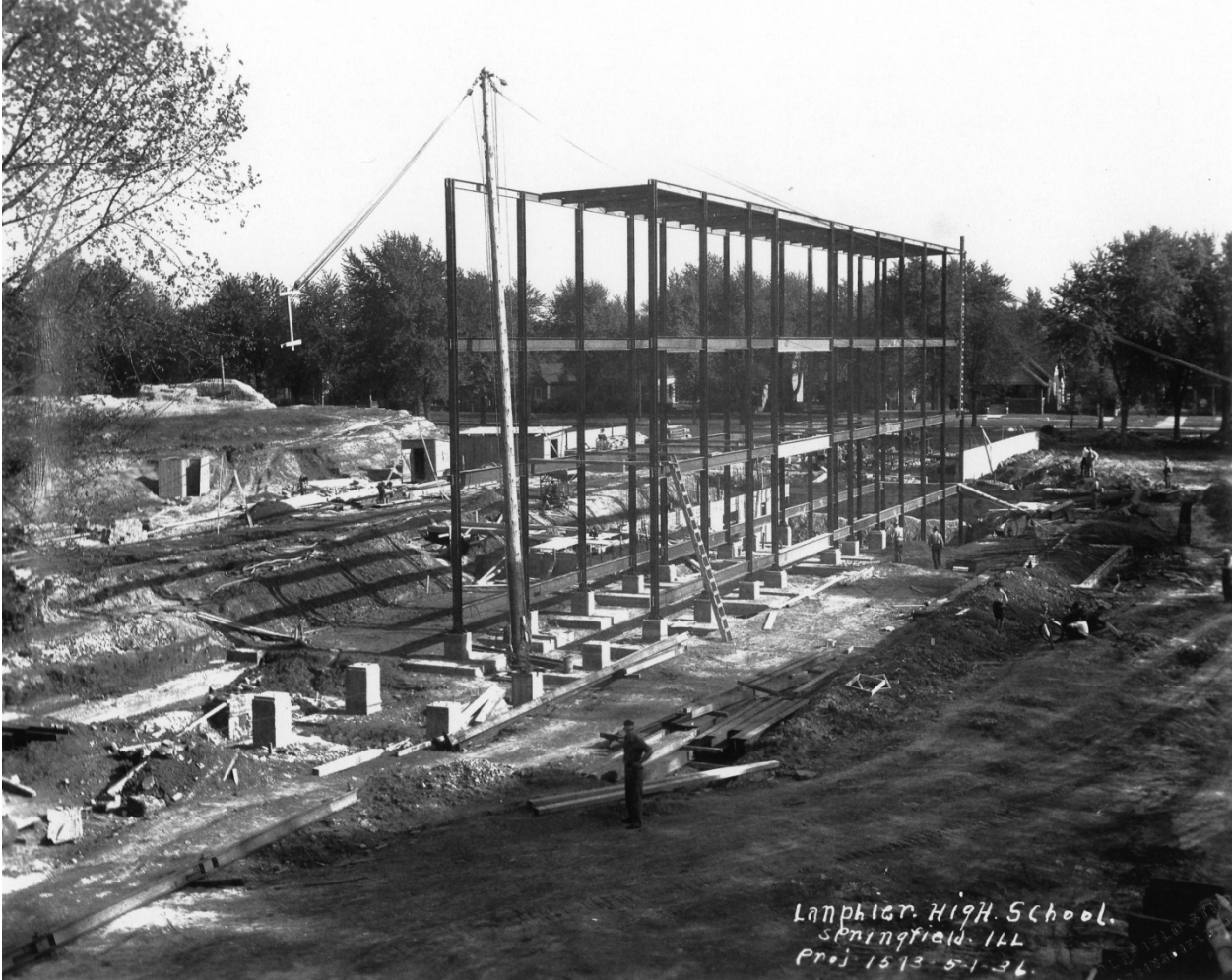
Lanphier High School construction, May 1, 1936. Photo courtesy Sangamon Valley Collection Lincoln Library.
