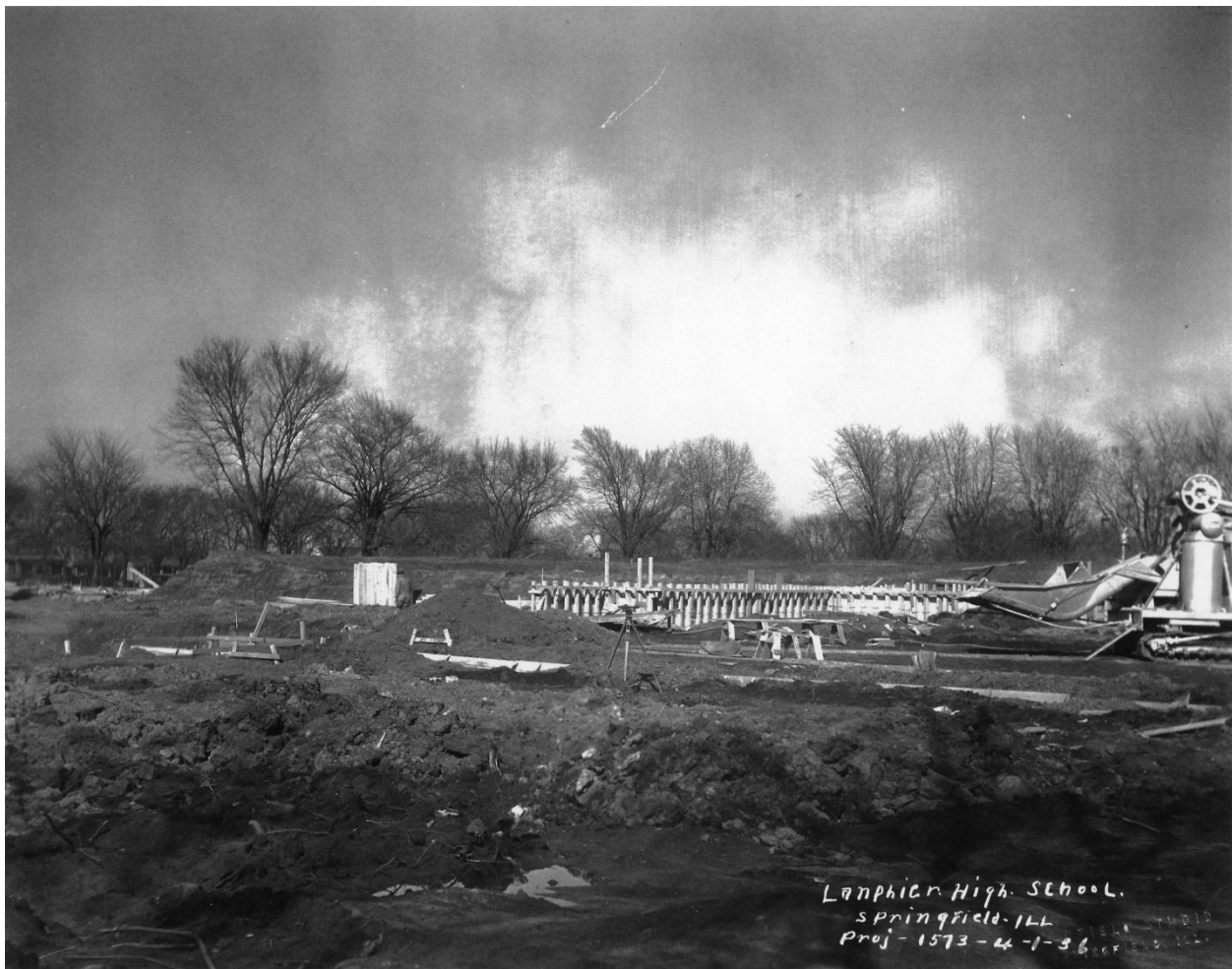
Lanphier High School construction, April 1, 1936. Photo courtesy Sangamon Valley Collection Lincoln Library.
